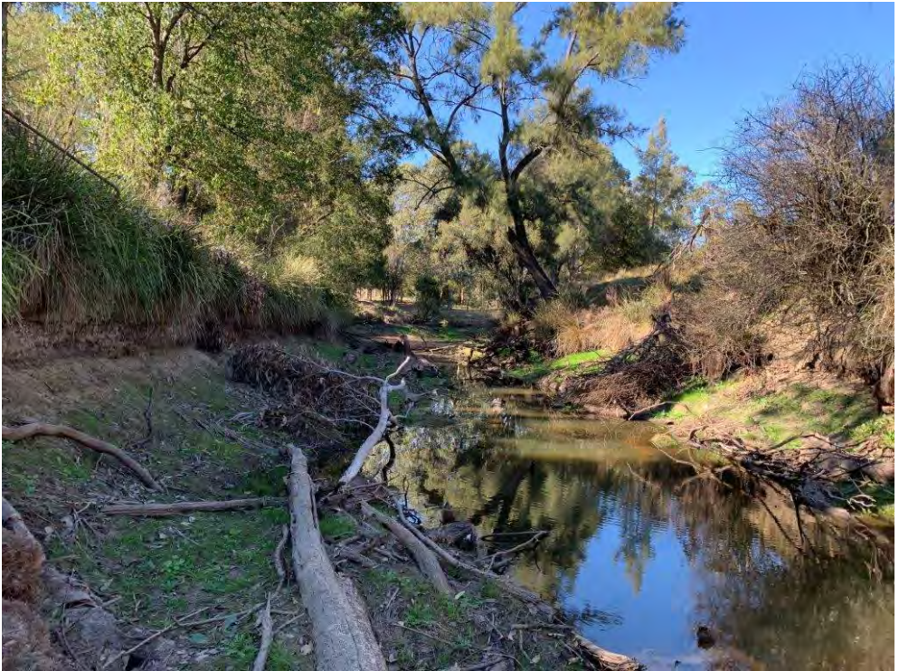
Photo 62 Avon River - Jacks Road crossing, site 121-04. Very poor bank condition, isolated pools with poor water quality
