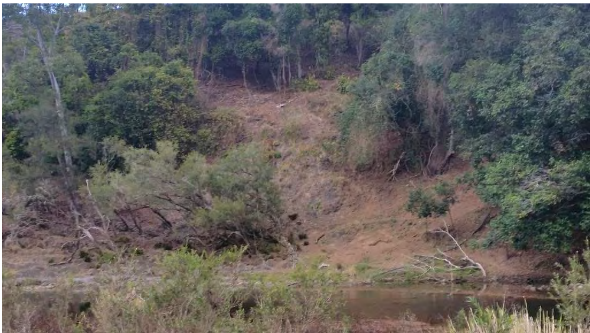
Photo 100 Manning River – site 105-1. Hillslope and bank erosion
