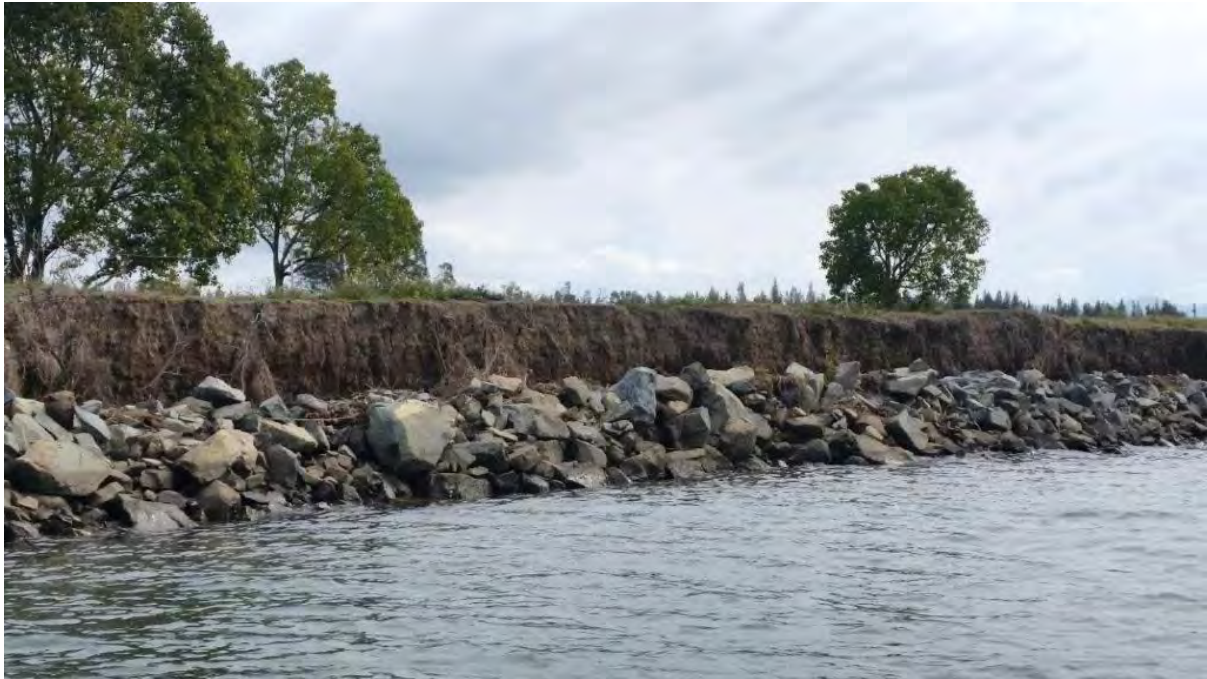
Photo 119 Manning River – Jones Is. subcatchment 205. Severe erosion of banks – rock revetment to reduce wash, further erosion.
