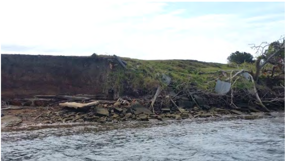
Photo 118 Manning River – Dumaresq Is. (subcatchment 208). Bank collapse, building/domestic waste along shoreline, possible attempt to prevent further erosion.
